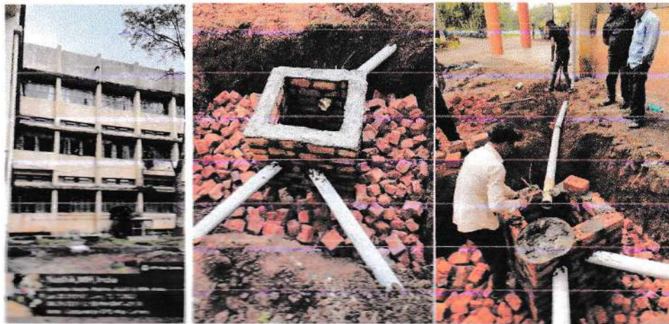
Rain Water Harvesting system
