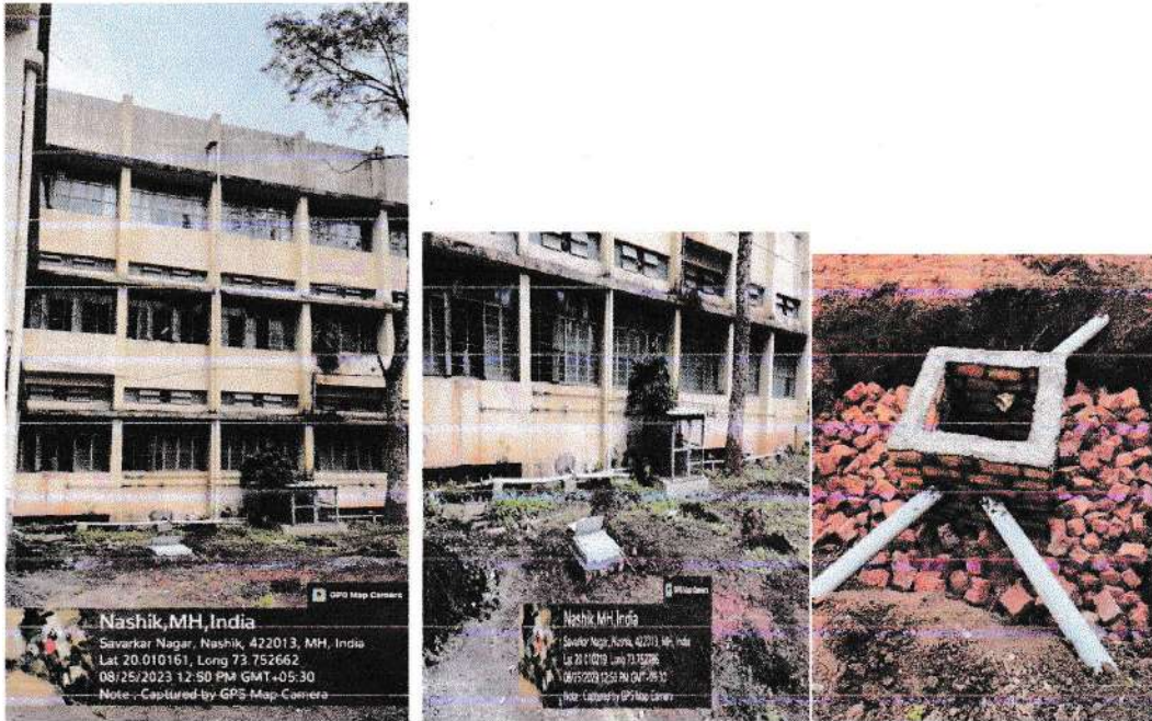
Rain water Harvesting system and recharge pit
