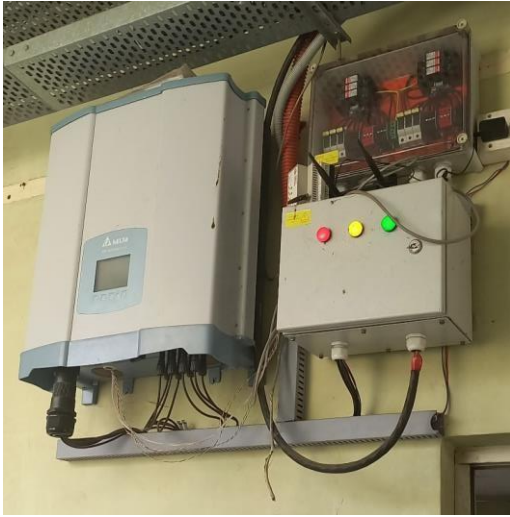
Solar Power System
