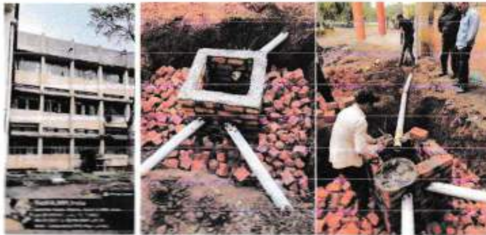
Rain Water Harvesting system
