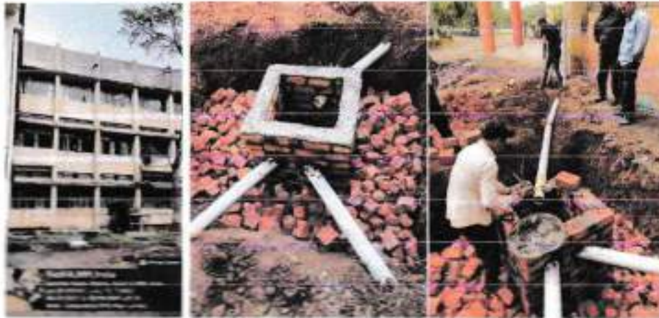
Rain Water Harvesting system
